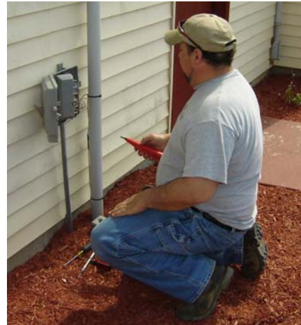
Mulberry Technician performing work during a service call.
